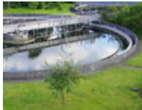
Sewage treatment plants
